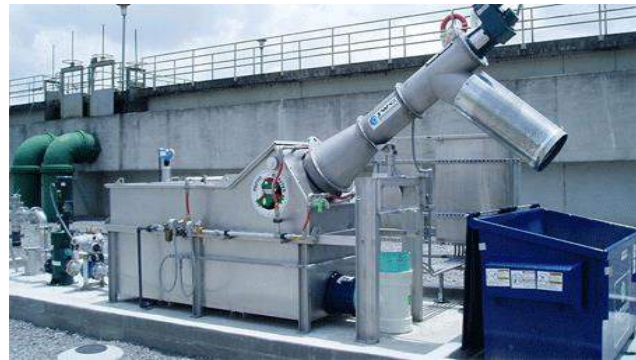
Figure 7-23: Septage Receiving Unit
