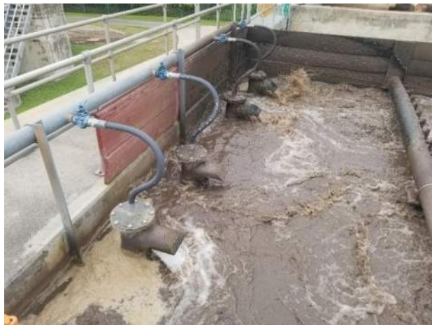
Figure 7-5: Aeration Basin Pumps
