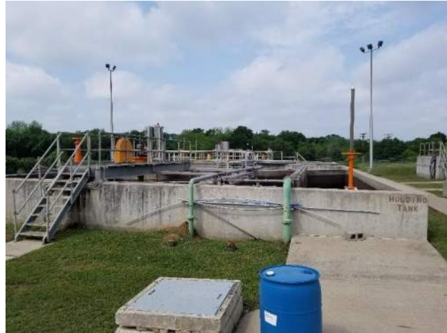
Figure 7-18: Sludge Holding Basin
