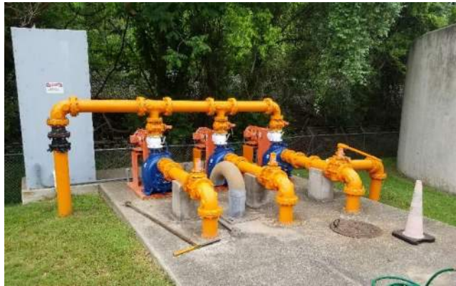
Figure 7-10: Drain Lift Station Pumps
