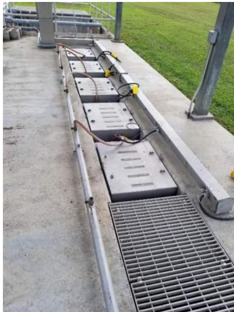
Figure 7-16: UV Disinfection Channels
