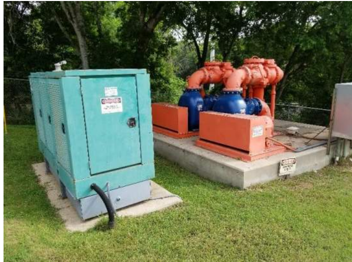
Figure 7-3: Generator & Relief Lift Station Pumps
