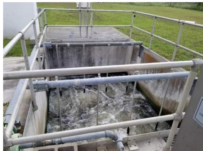
Figure 7-17: Post Aeration Basin and Outlet Box
