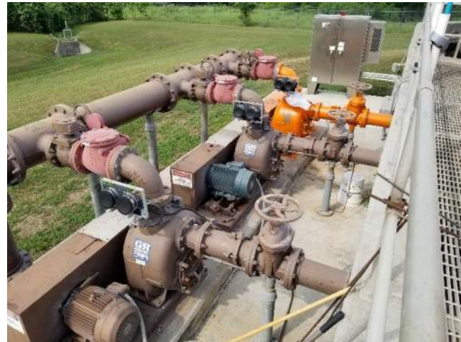
Figure 7-15: RAS Pump Station
