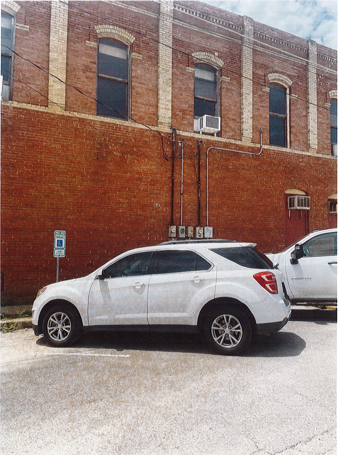
- Existing electrical panels -
